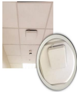
Sample of an RFiD reader, these are most frequently hidden behind ceiling tiles
